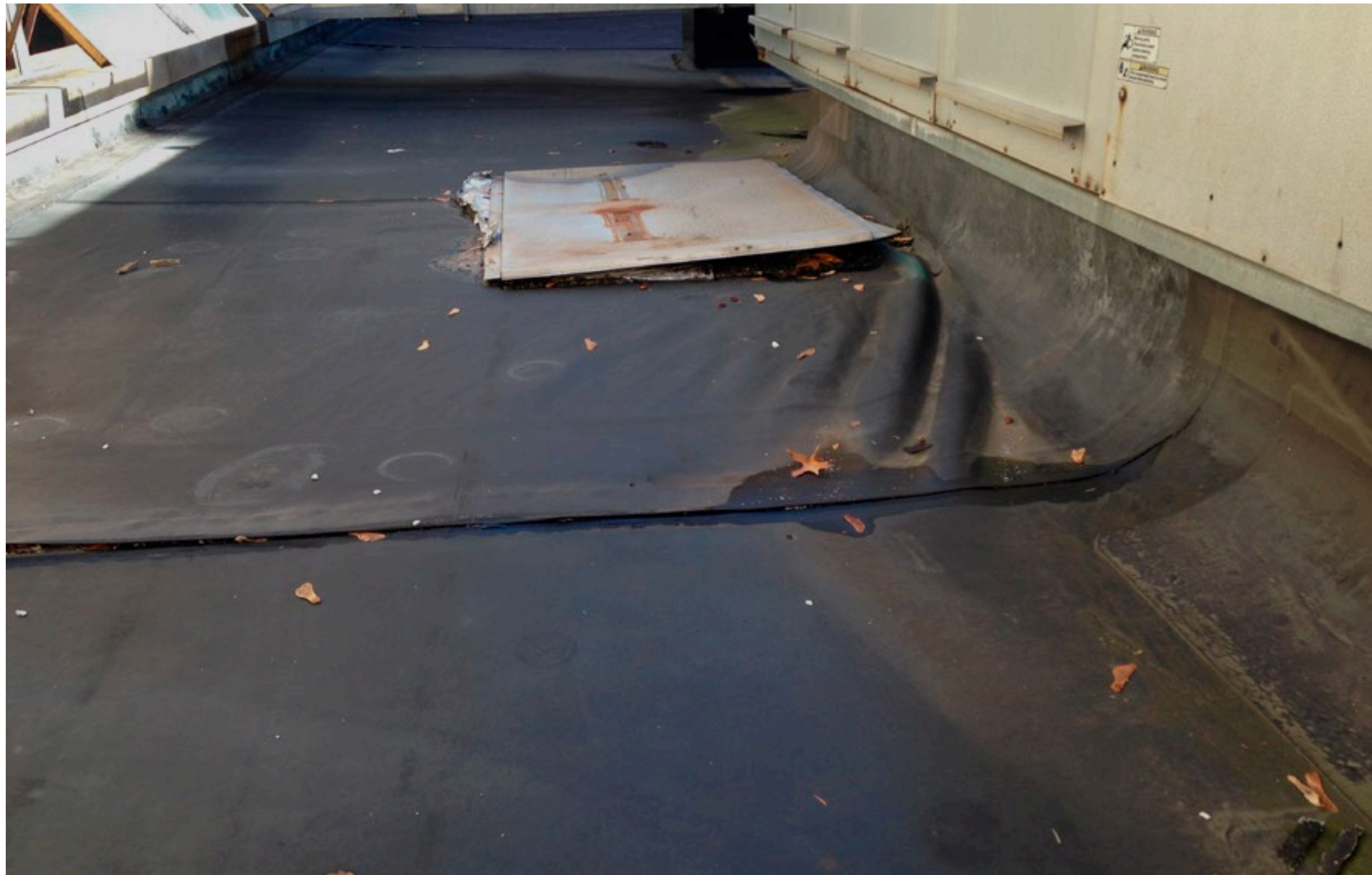
DETERIORATED ROOF SECTION - SYSTEM NO LONGER ADHERED, WATER MAY HAVE DEVELOPED BELOW THE MEMBRANE
