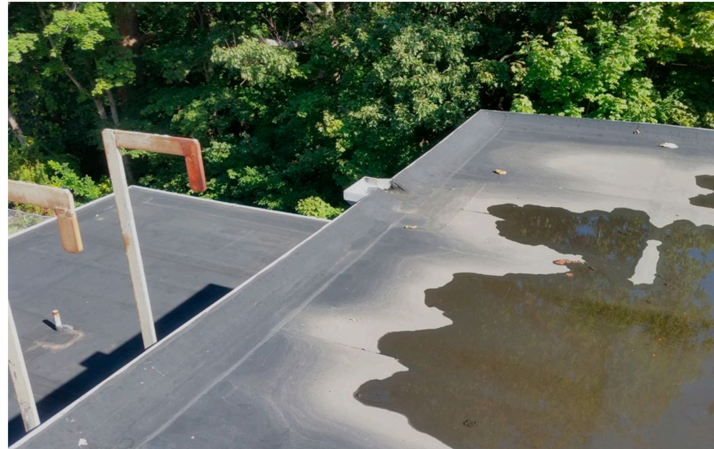
WATER REMAINING ON ROOF DAYS AFTER RAIN EVENT
