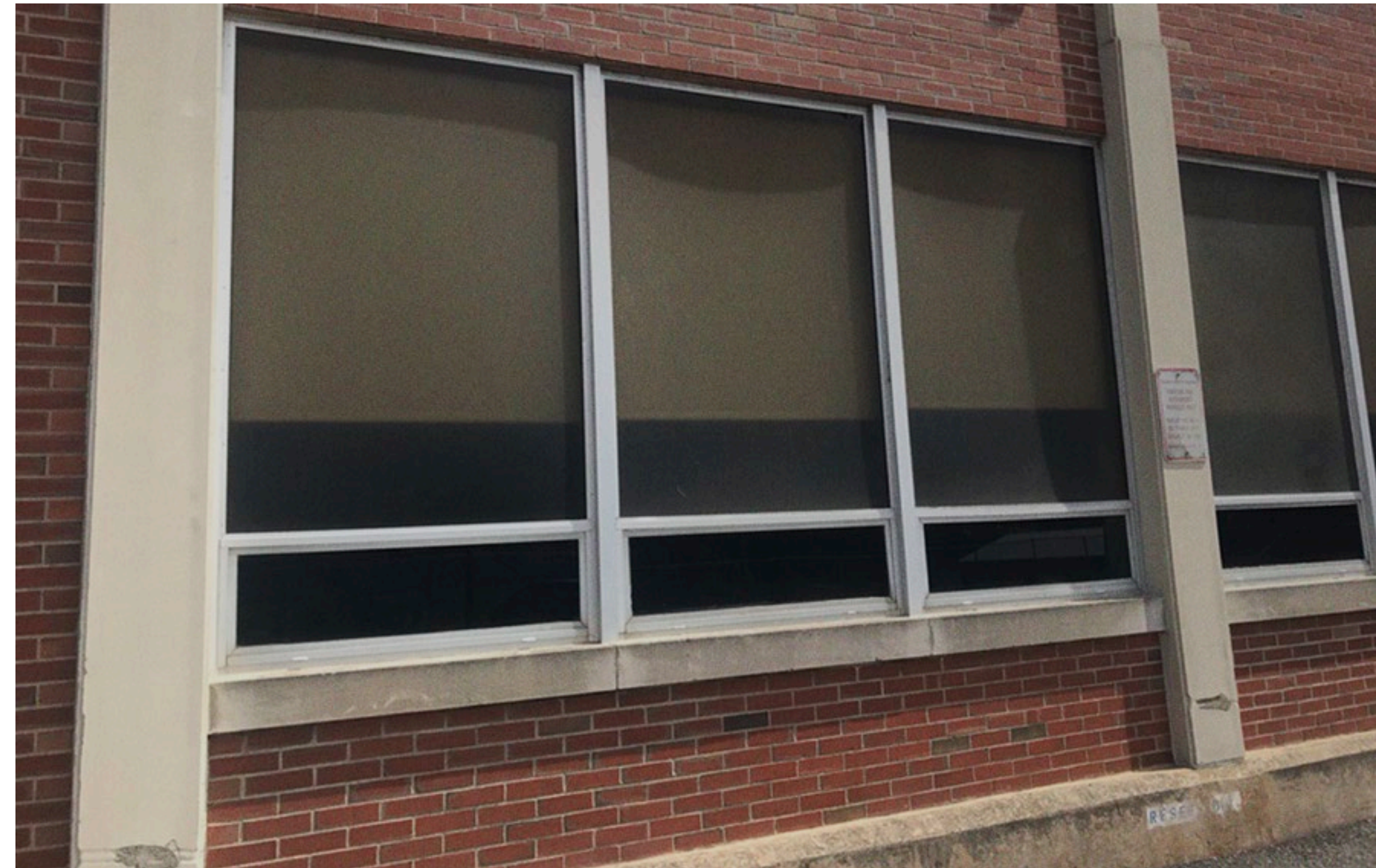
EXISTING WINDOWS ARE SINGLE PANE AND INEFFICIENT
