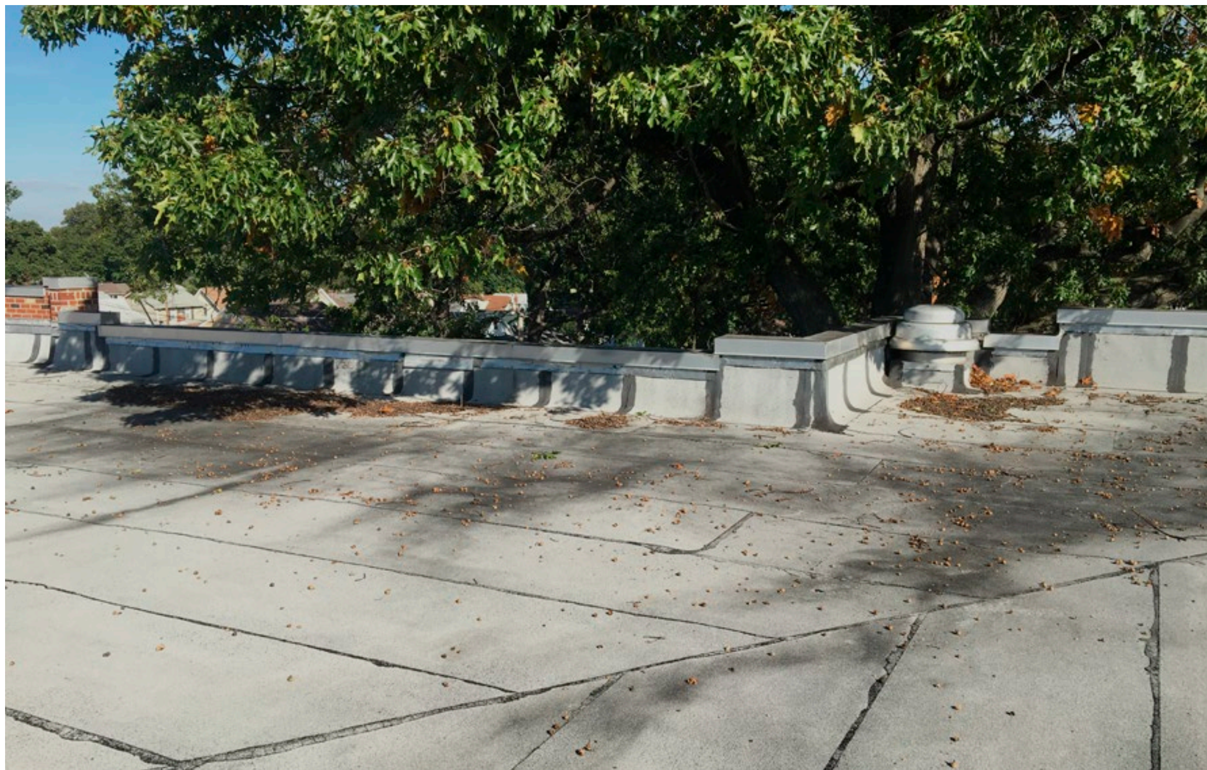
DETERIORATED ROOF SECTION - DARK AREAS INDICATE STANDING WATER
