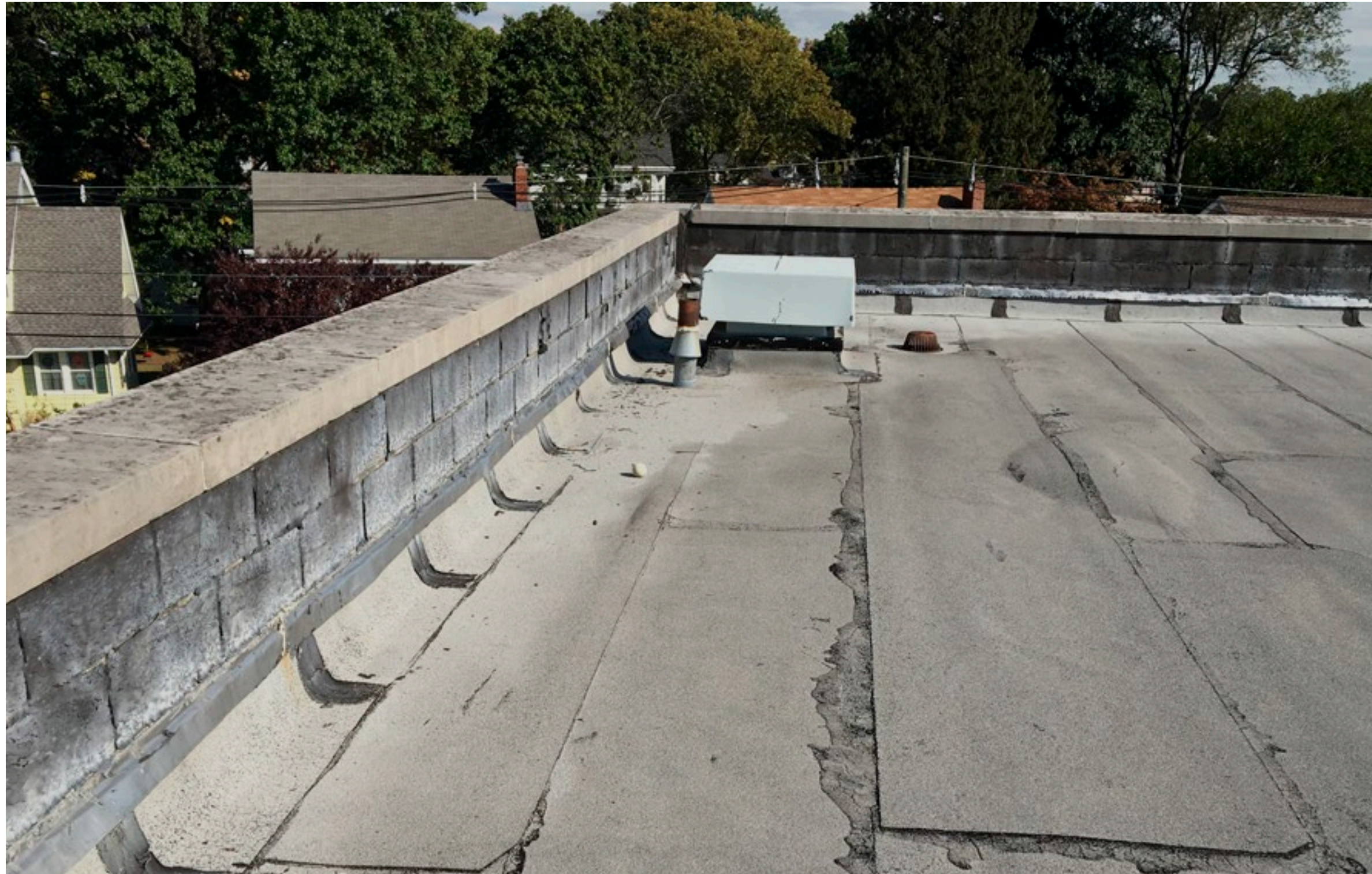
DETERIORATED ROOF SECTION - VISIBLE AIR BLISTERS, POOR FLASHING AND COPING
