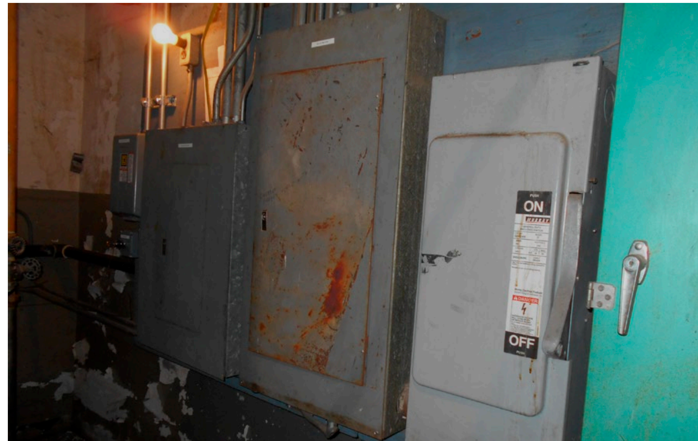
RUSTED ELECTRICAL PANELS
