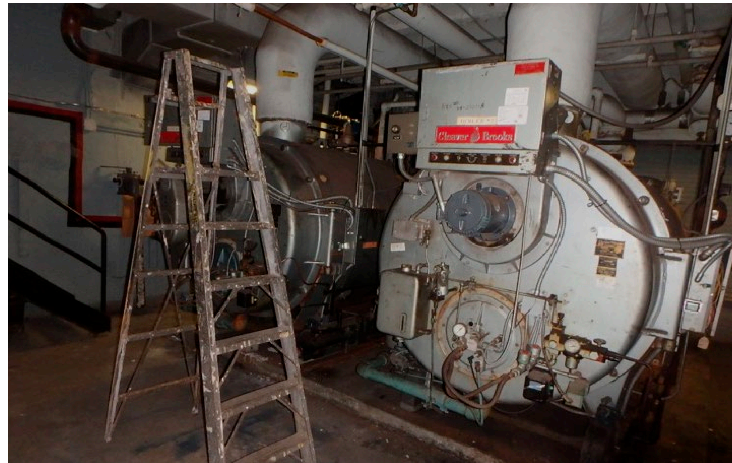
BOILER ROOM CONTAINS ASBESTOS ON PIPING
