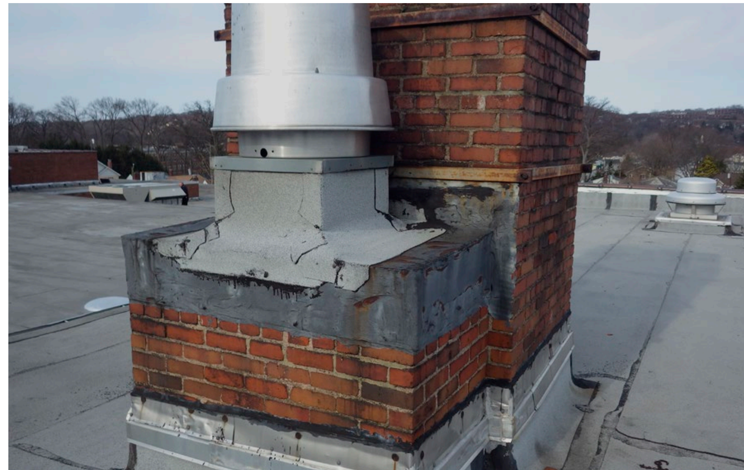
CHIMNEY FLASHING IN POOR CONDITION
