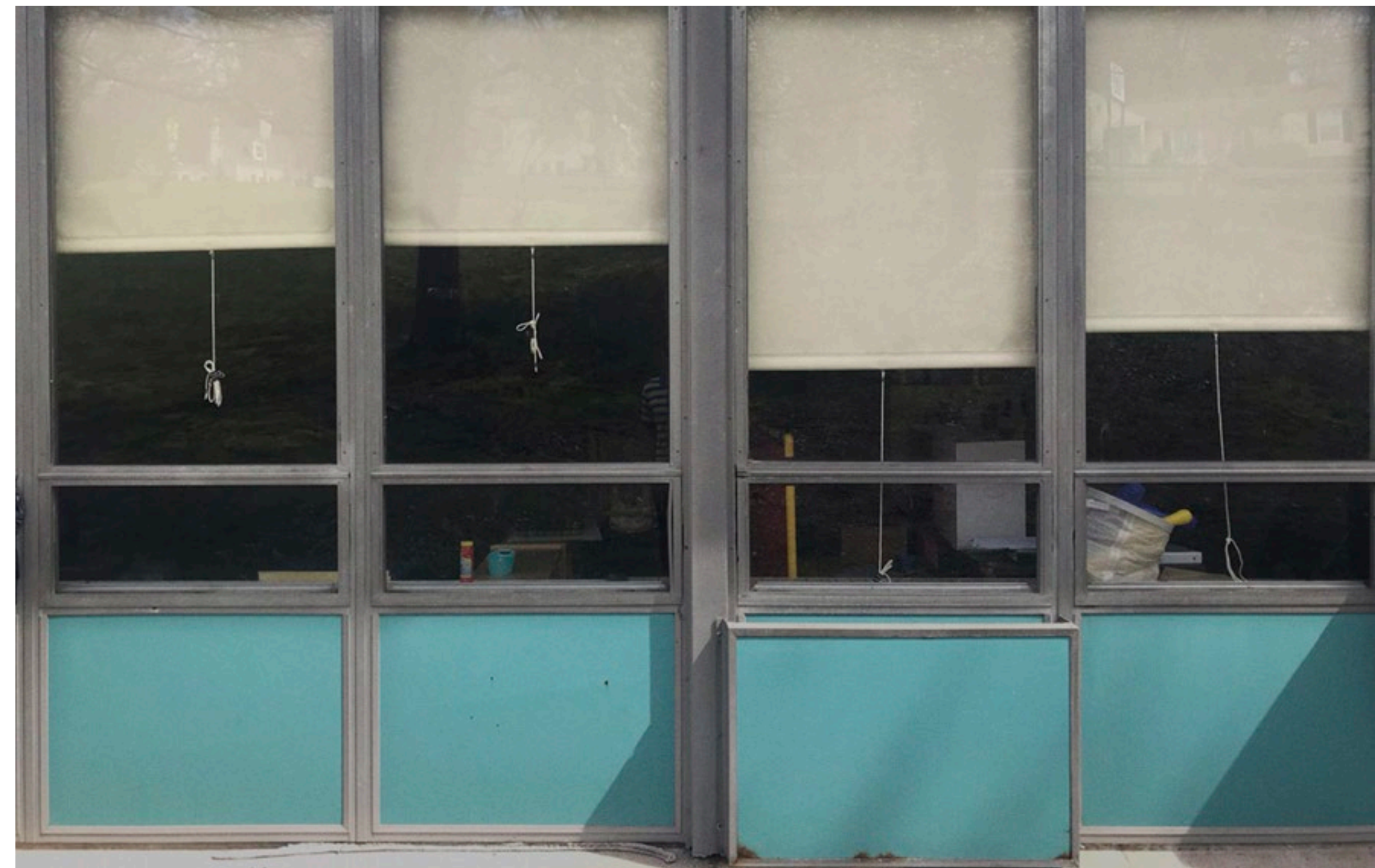
EXISTING CURTAIN WALL SYSTEMS ARE SINGLE PANE AND INEFFICIENT; PANELS ARE BEGINNING TO RUST OUT
