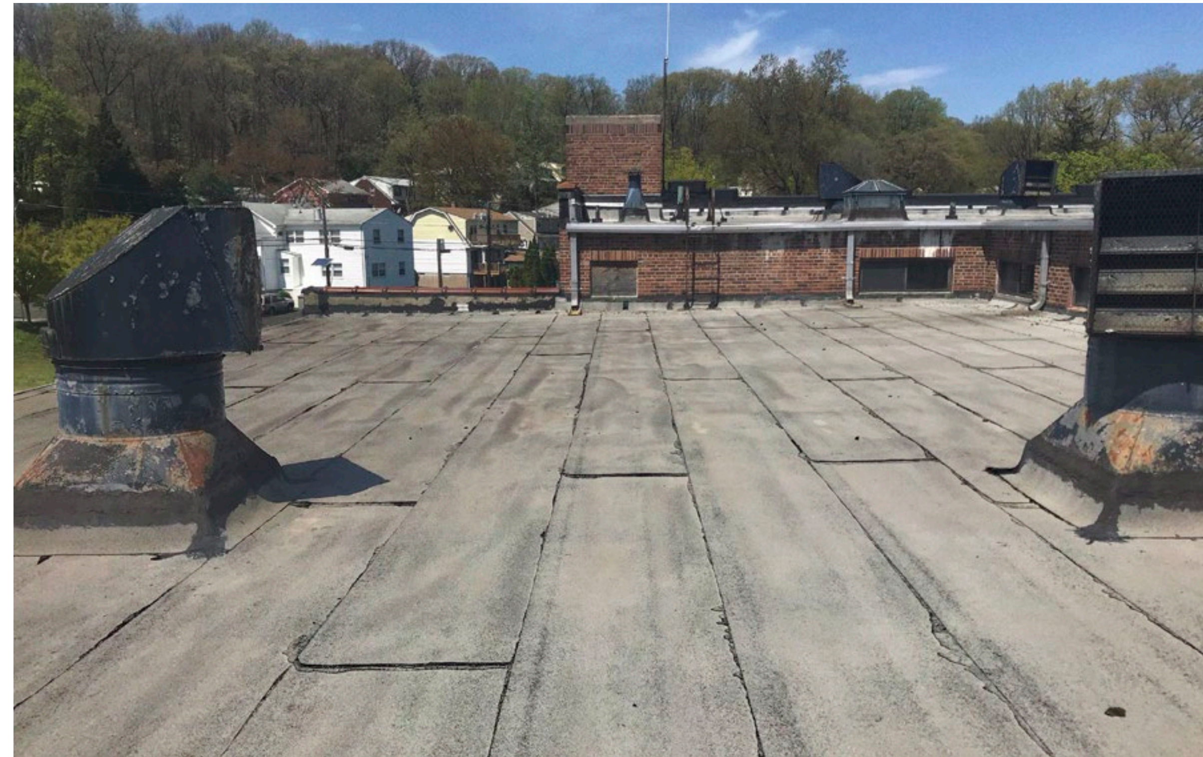
AGED ROOF MEMBRANE IN POOR CONDITION
