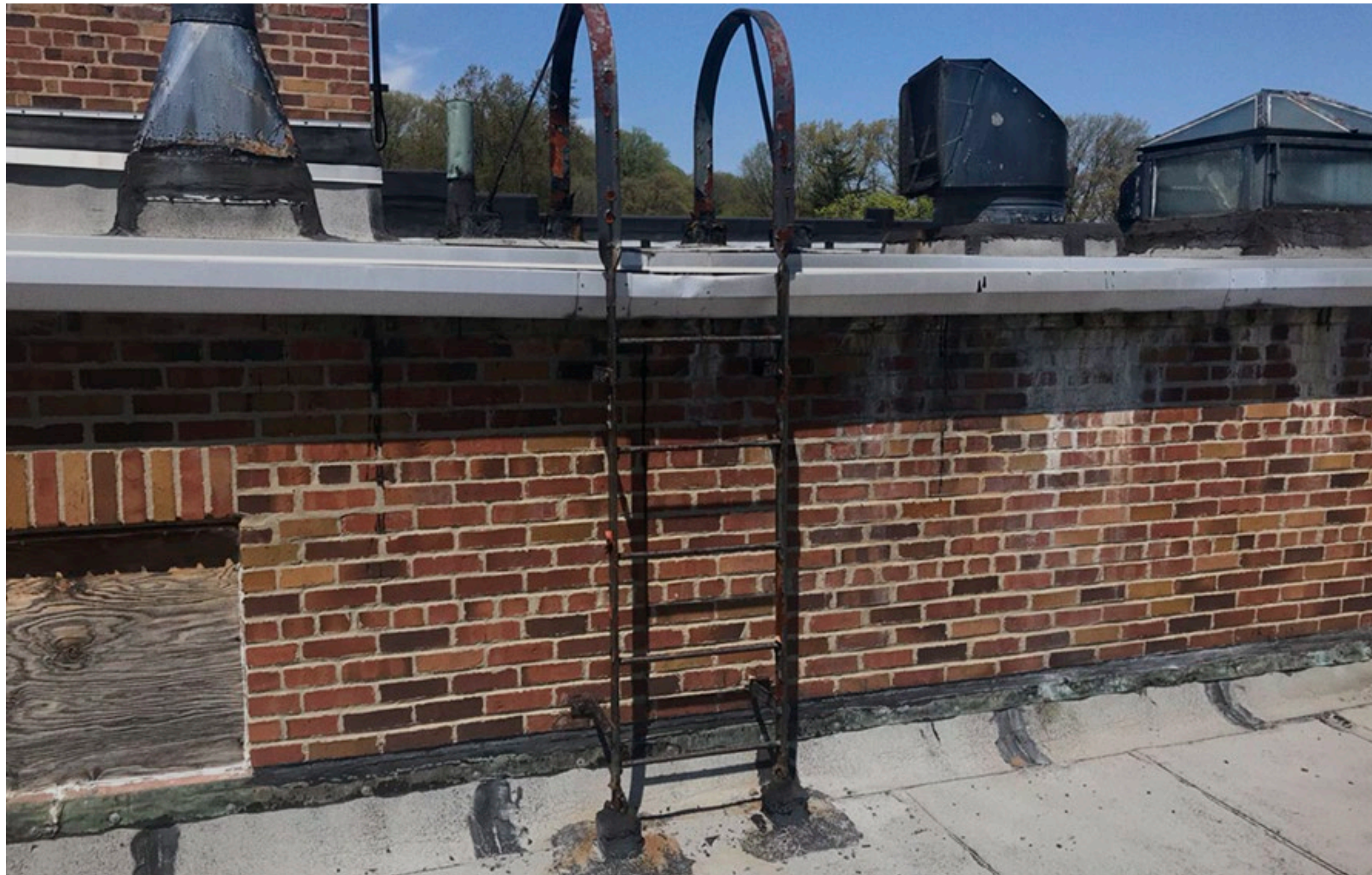
ROOF FLASHING HAS BEEN REPAIRED MULTIPLE TIMES; EFFLORESCENCE ON MASONRY WALL IS INDICATION OF WATER PENETRATION FROM ABOVE
