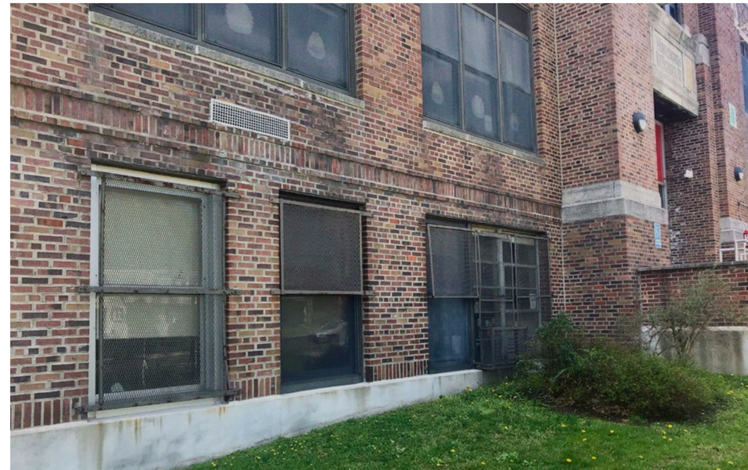
EXISTING WINDOWS ARE SINGLE PANE AND INEFFICIENT
