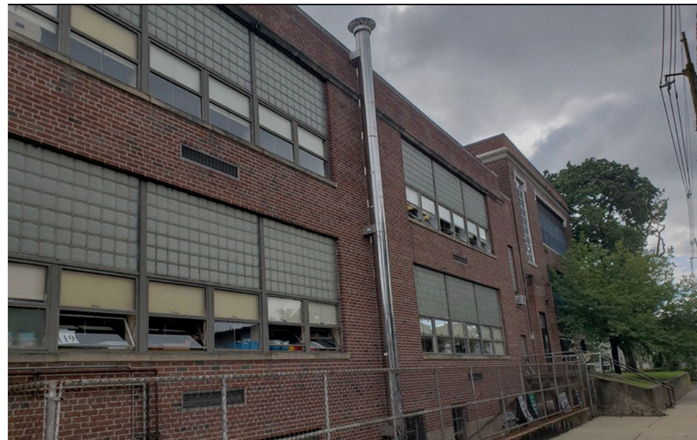
EXISTING WINDOW SYSTEM IS SINGLE PANE AND INEFFICIENT
