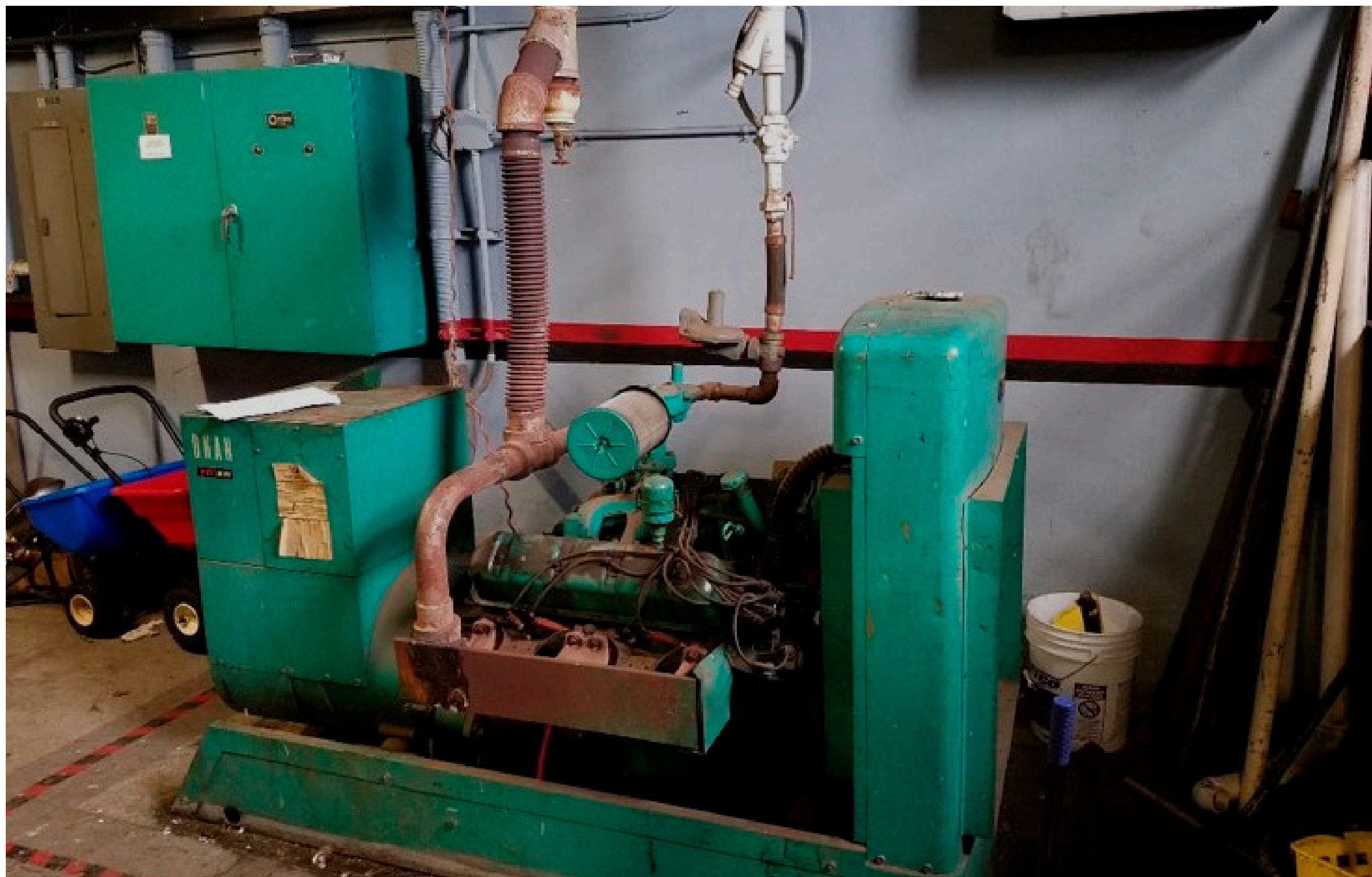
EXISTING GENERATOR IS WELL BEYOND IT'S LIFE EXPECTANCY
