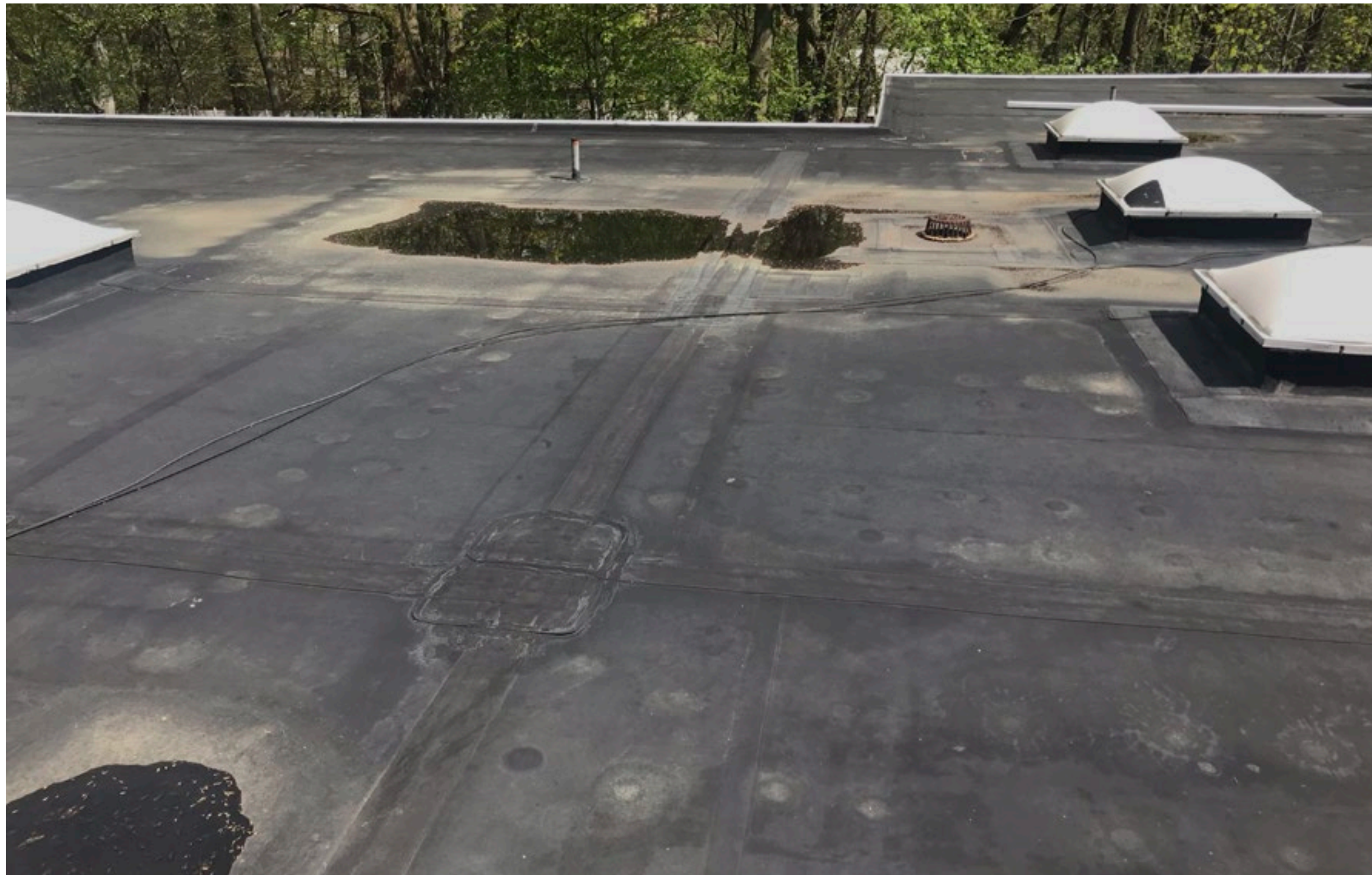
DETERIORATED ROOF SECTION - RETAINING WATER AND, NOT DRAINING PROPERLY
