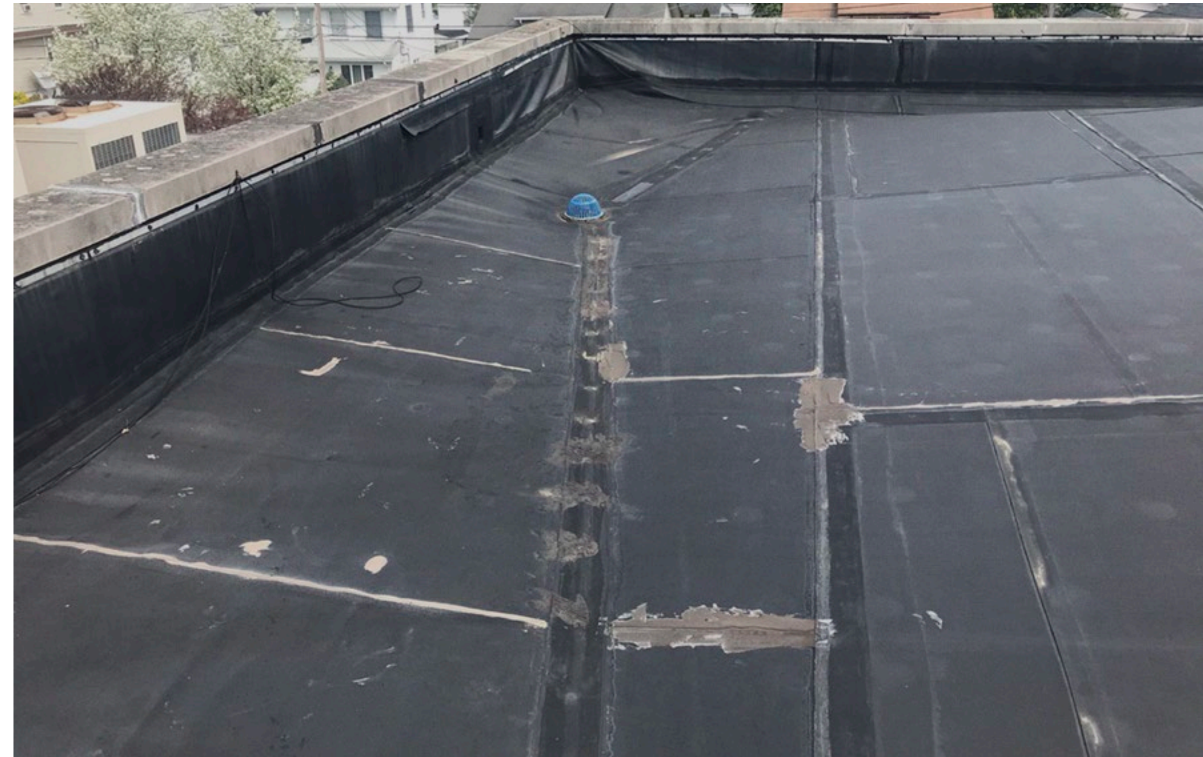
DETERIORATED ROOF SECTION - DELAMINATIONS OF ROOF MEMBRANE; PATCHWORK OF SEAMS THROUGHOUT
