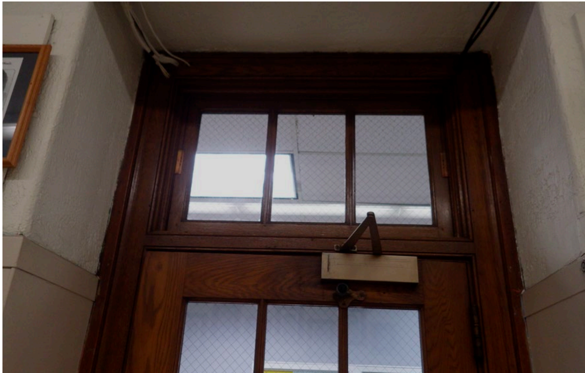
GLASS ON DOOR CANNOT BE SECURED DURING LOCKDOWN; DOORS DO NOT MEET CURRENT CODE
