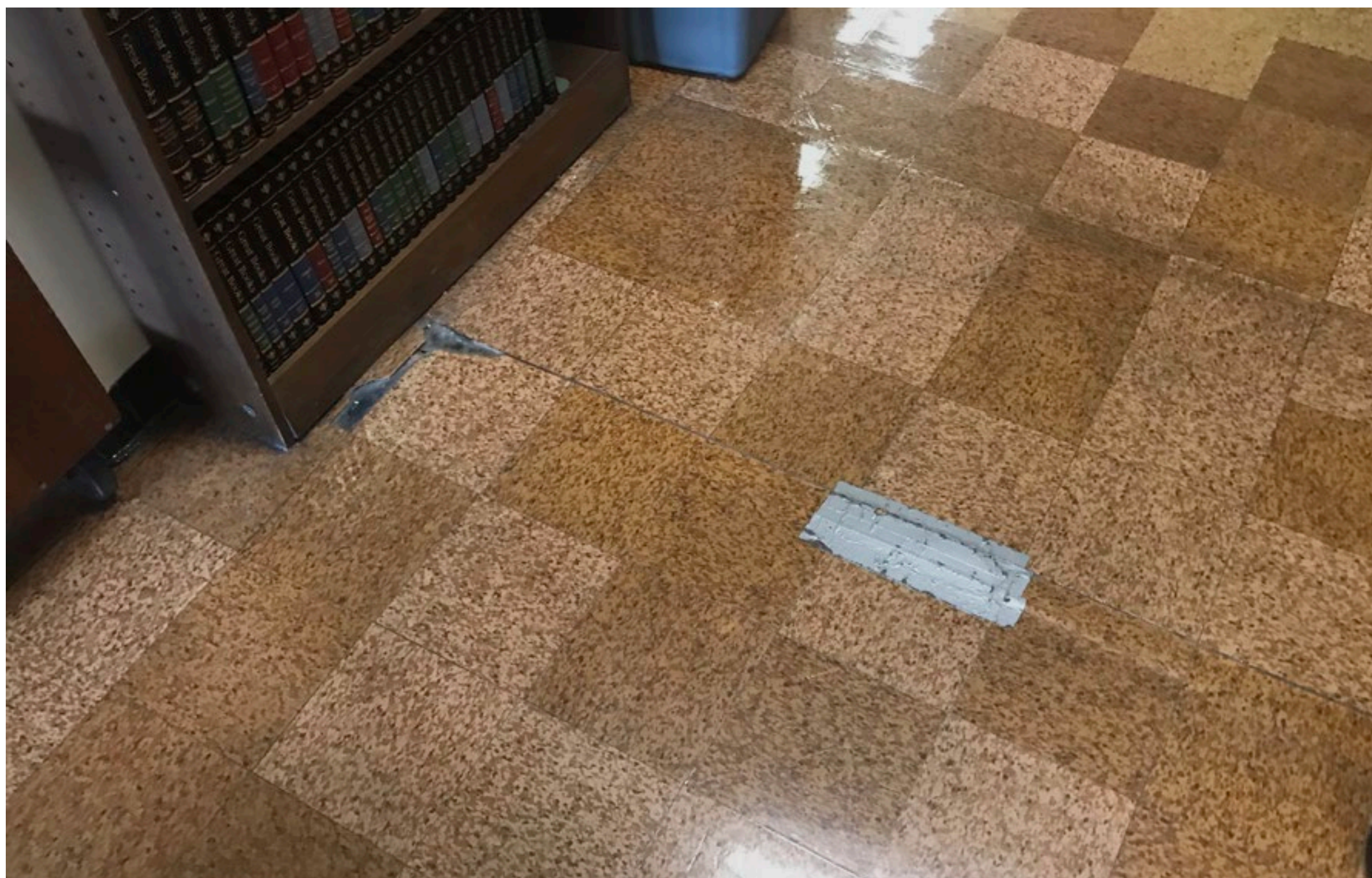
MEDIA CENTER FLOORING- CRACKING & POPPING 9X9 FLOOR TILES
