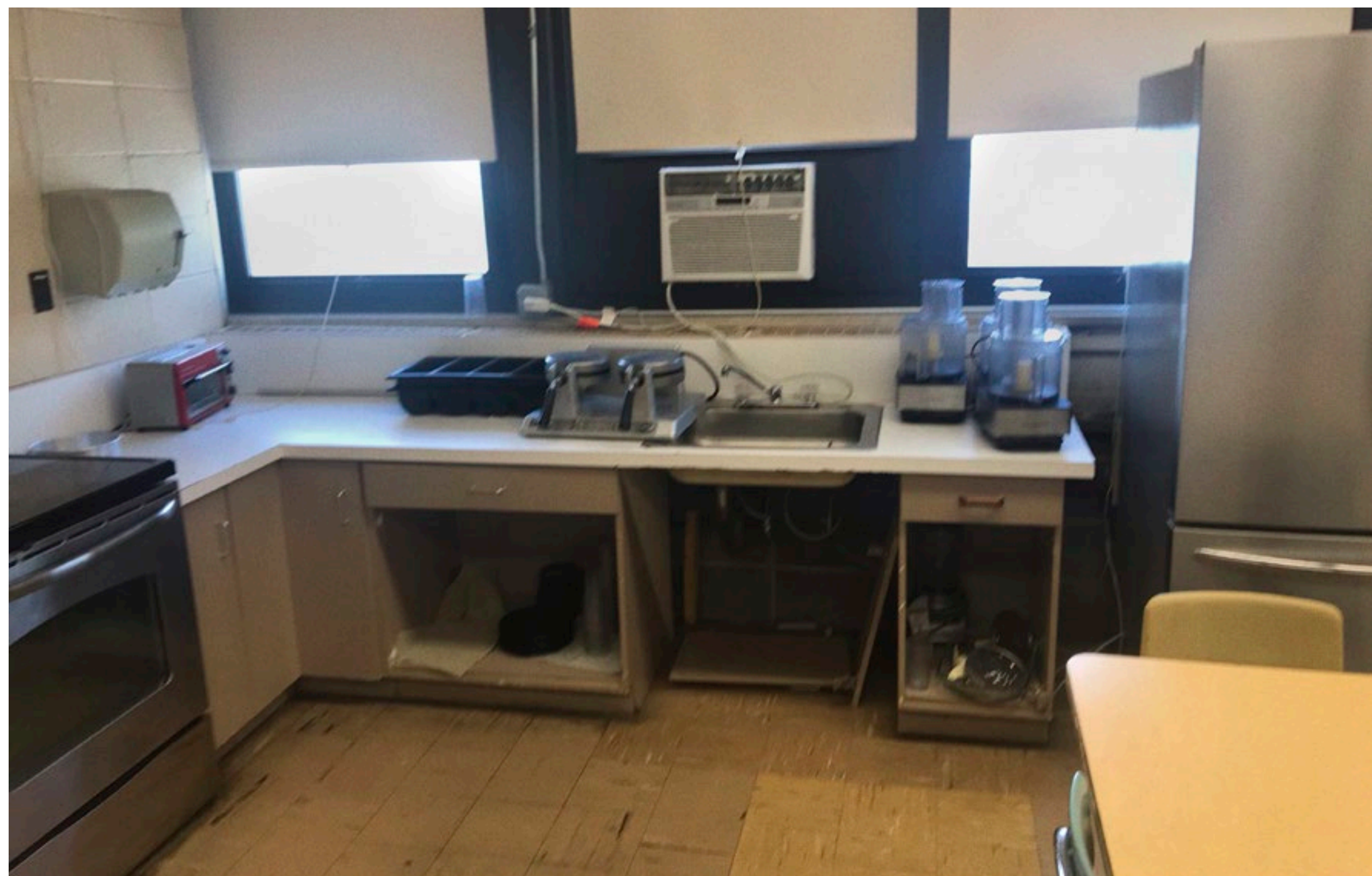
CULINARY ARTS WORKSTATION- DETERIORATING CASE WORK, COUNTERTOP, FLOORING & POOR LIGHTING
