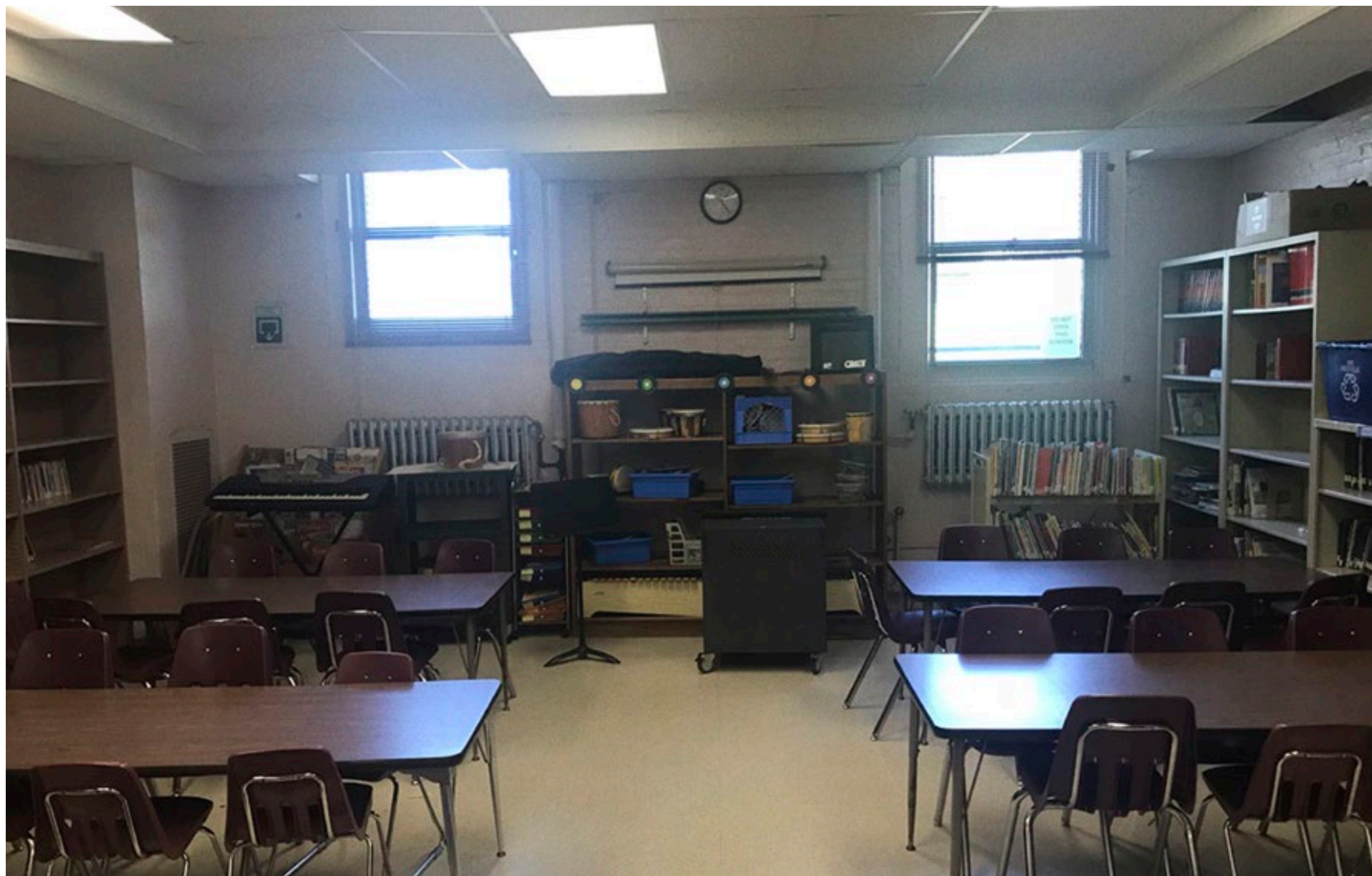
MEDIA CENTER – BOWING CEILING TILES; AGED INSUFFICIENT METAL CASEWORK
