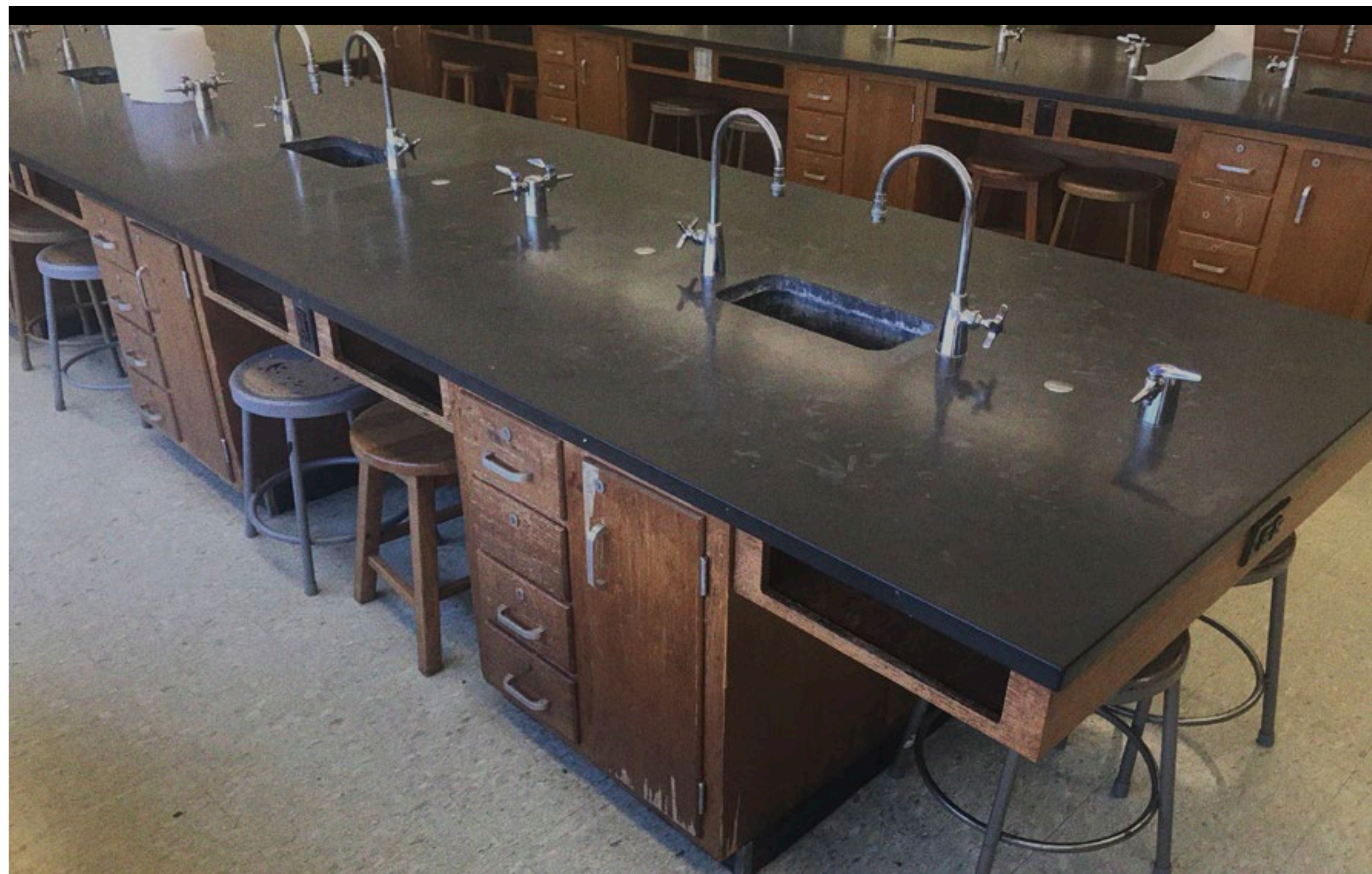
SCIENCE LABS- ORIGINAL FIXED, INFLEXIBLE DETERIORATING WORKSTATIONS AND CASEWORK; MISSING DRAWERS & HARDWARE
